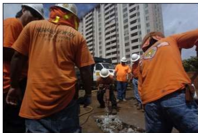
Construction workers with Henkels and McCoy Inc. removed old concrete last week to make way for a new playground foundation at Kuhio Park Terrace. The state's largest public housing project has not had a playground in its 40 years.
